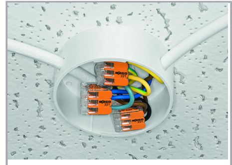
Lighting distribution in a ceiling canopy
