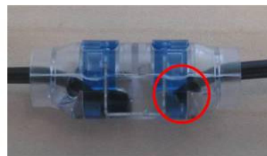
Wires terminated incorrectly
